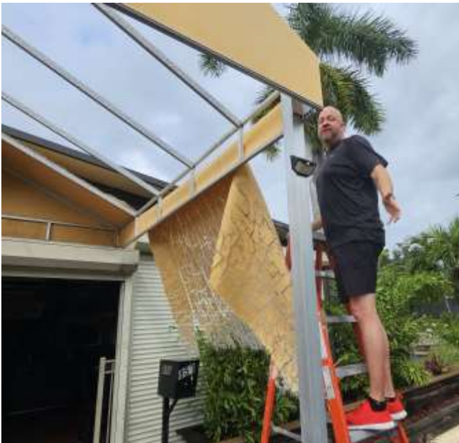
Member and Goombah co-owner Mike helps remove canopy damaged in the storm.
